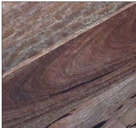
The photo to the left shows circular swirl marks that are visible under down light. The photo to the right shows the same section of floor in natural light without the down lights on and the swirl marks are not visible.
